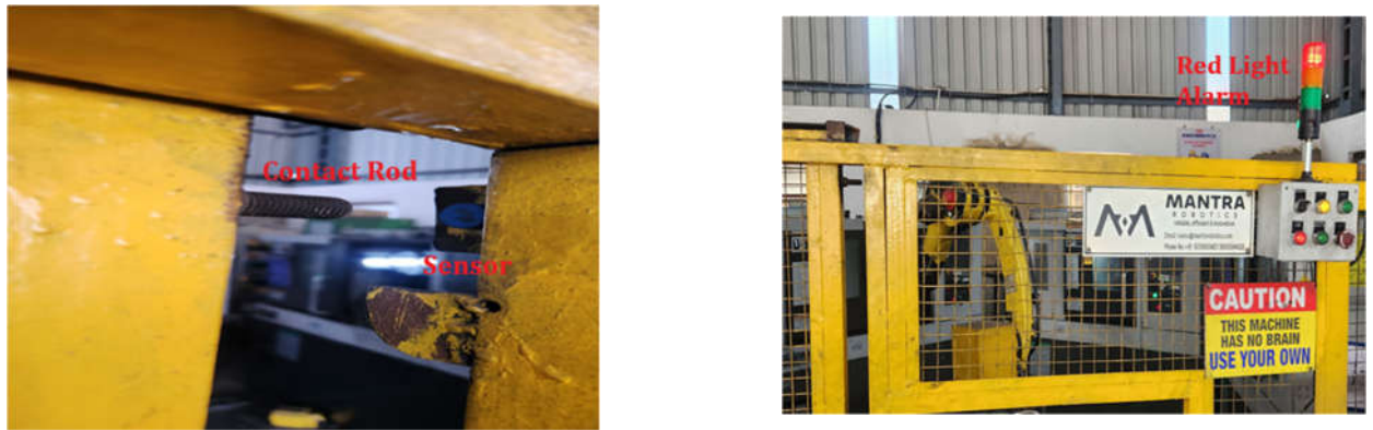
Fig. 6 Contact type Poka Yoka used for robot cell door. After door open steel rod contact lose with sensor and red light C alarm start and robot movement stop.
